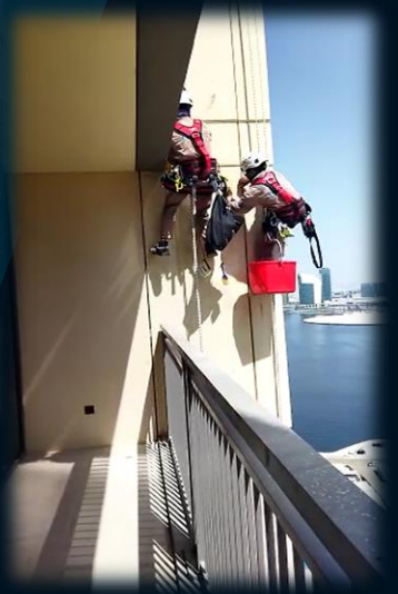
Client: EMAAR DEVELOPMENT P.J.S.C. Project Name: Creek Rise Tower 1 & 2 Scope of Work: GRC Paint Removal & External Façade Glass Cleaning
